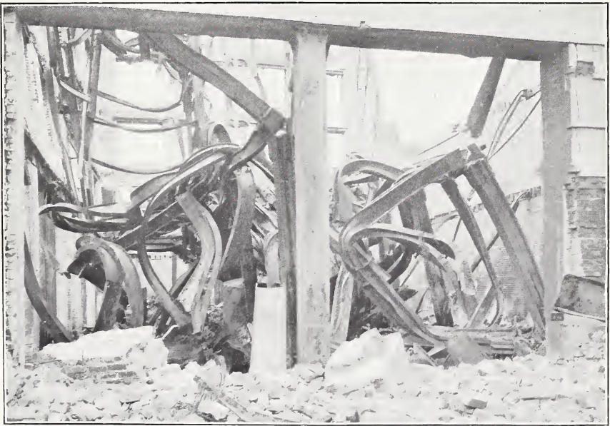
B. UNPROTECTED STEEL FRAME AND GENERAL FLIMSY CONSTRUCTION, COWELL BUILDING.
